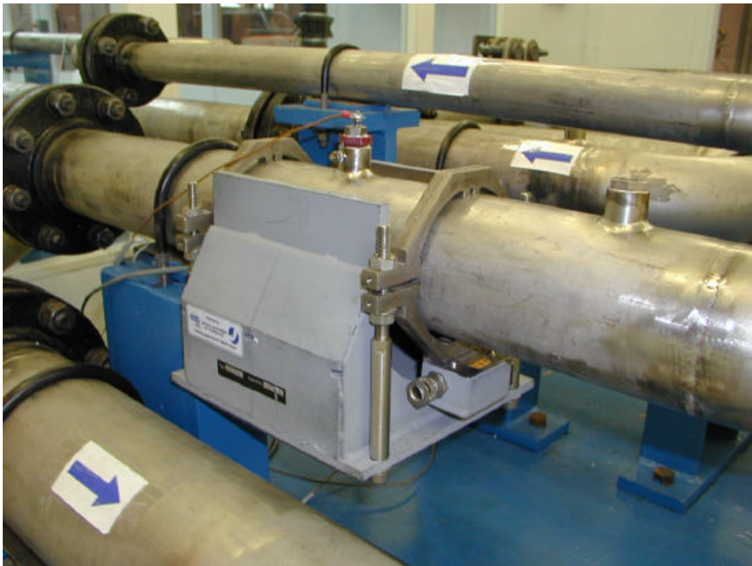
Figure 2. EM flow meter installed on a 4-inch supply line.
